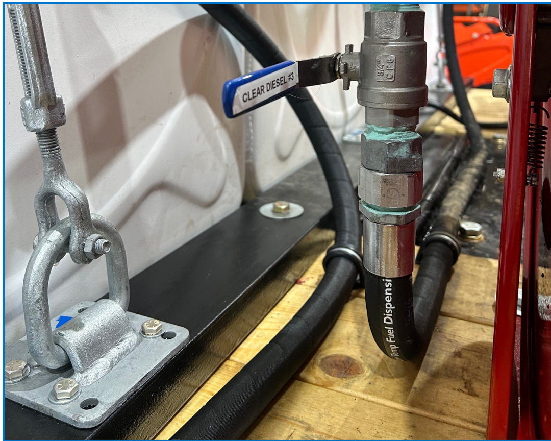
Image 2.0 - Image - Tanks Anchors Bolted to C-Channel & C-Channel Connection to Deck
