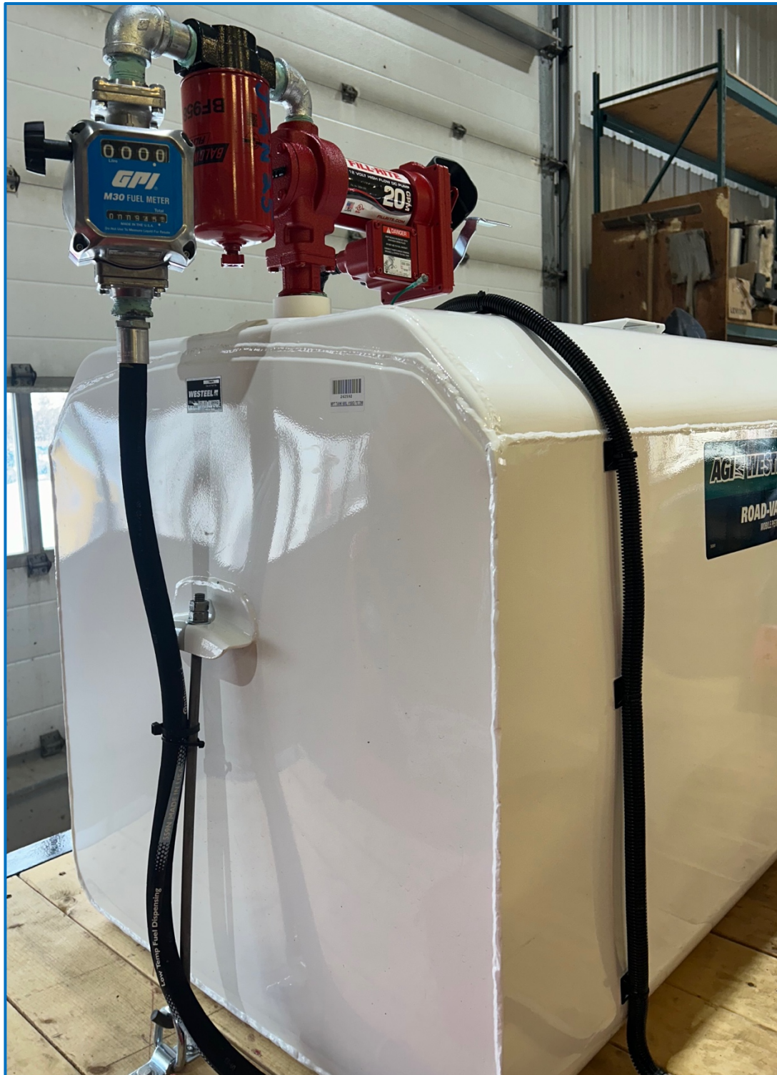
Image 4.0 - Image showing the electrical wiring (Sheathing)
