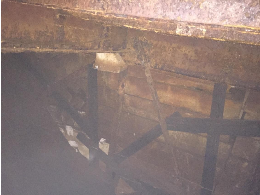
Figure 6 - View inside Void A, showing the foam installed in the inboard portion of the space
