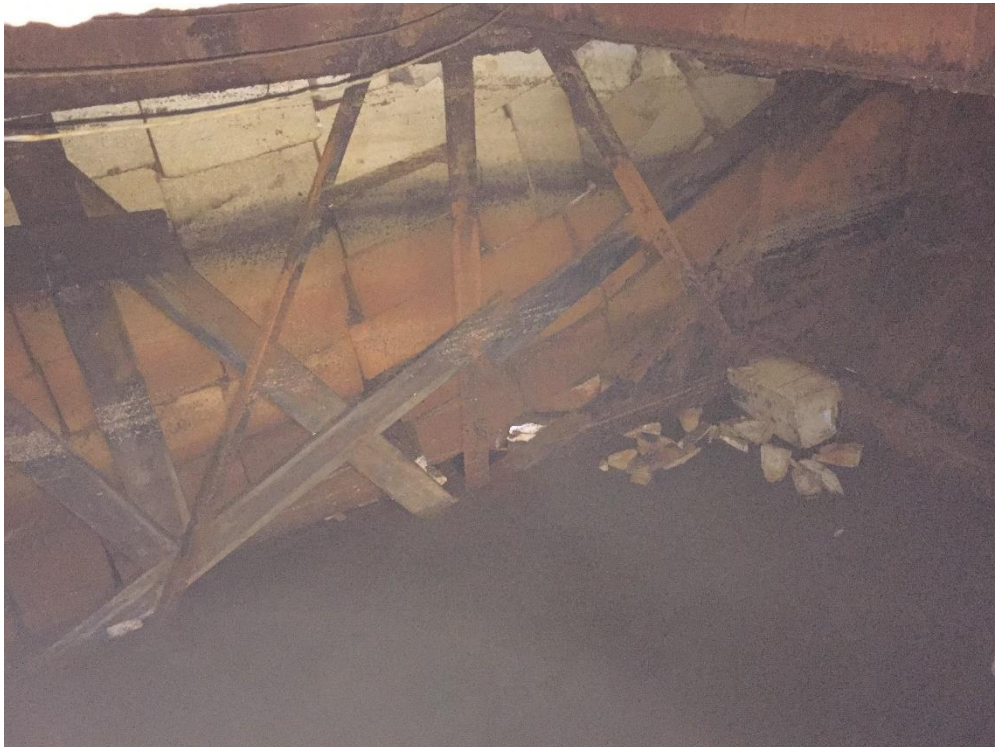
Figure 7 - View inside Void F, showing the foam installed in the inboard portion of the space
