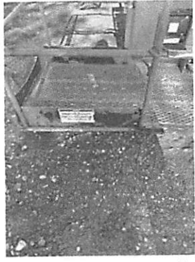
P9.2: Crushed bottom rail
