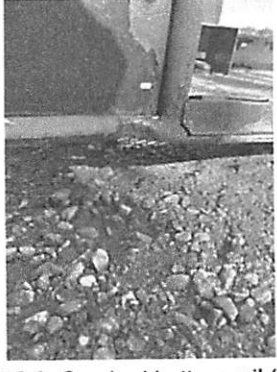
P9.3: Crushed bottom rail (close up)
