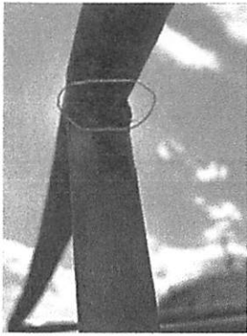
P9.5: Repair check: incomplete weld on basket top rail. No fusion.
