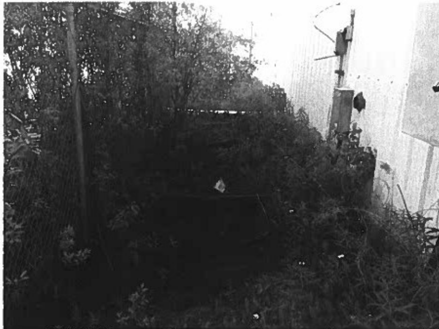
Photo 16: View of the staining behind the building facing east (Area 2).
