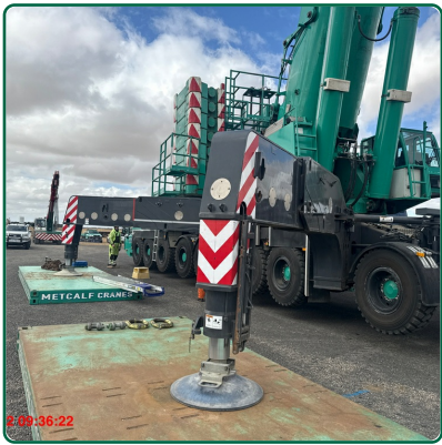
Outrigger Hazard Striping
