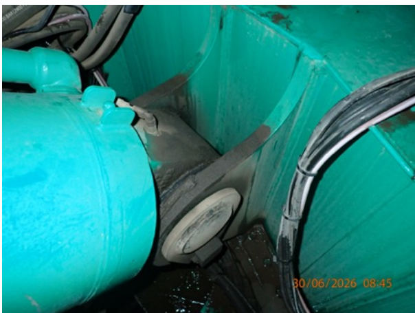
Photo 13: Lowe luffing cylinder weld & mount
