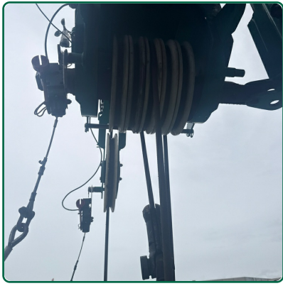
Head Sheaves and bearings
