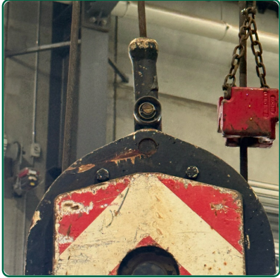
Main Hoist Rope Socket and Pins
