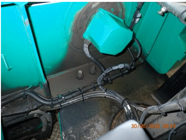
Photo 11: Counterweight mount welds
