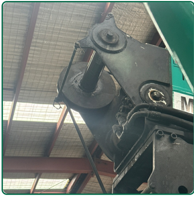
Idler Sheave and Bearing
