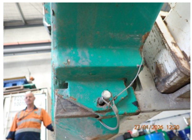
Photo 20: Counterweight-spreader bar mount
