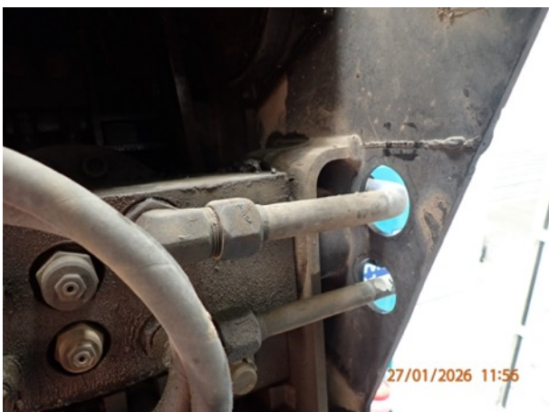
Photo 7: Telescoping cylinder & sheave mount
