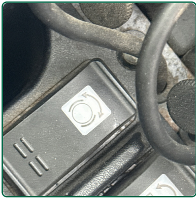
Slew Brake Checked and working satisfactory at the time of inspection
