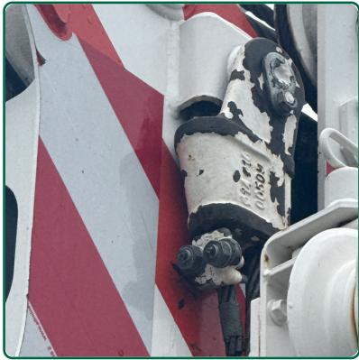
Main Hoist Rope Socket and Pins
