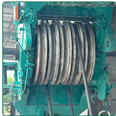
Head Sheaves and bearings
