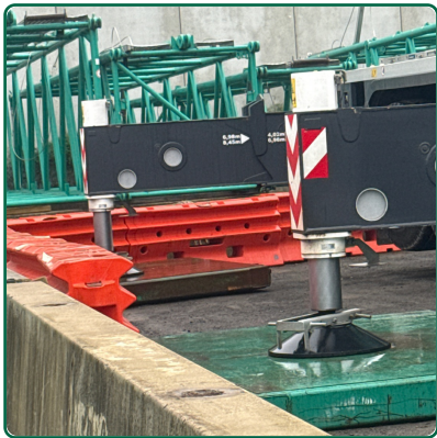
Outrigger Hazard Striping
