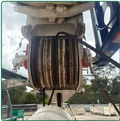
Head Sheaves and bearings
