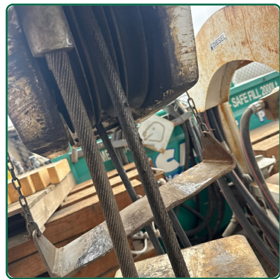
Head Sheaves and bearings
