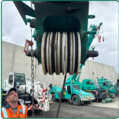
Head Sheaves and bearings
