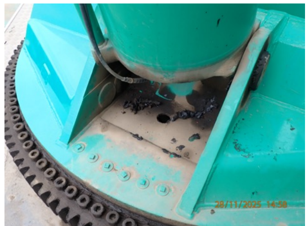
Photo 10: Lower luffing cylinder mount
