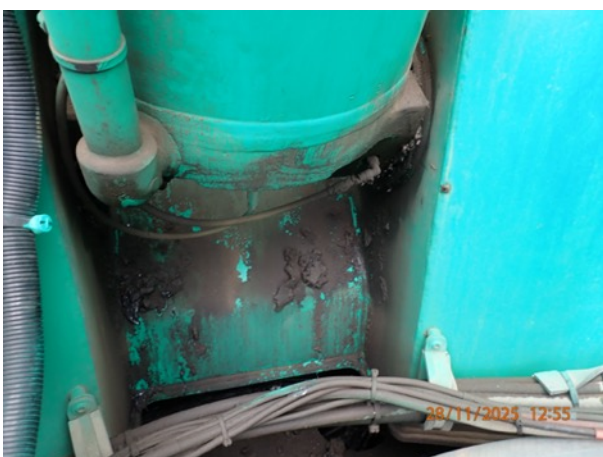
Photo 7: Lower luffing cylinder mount
