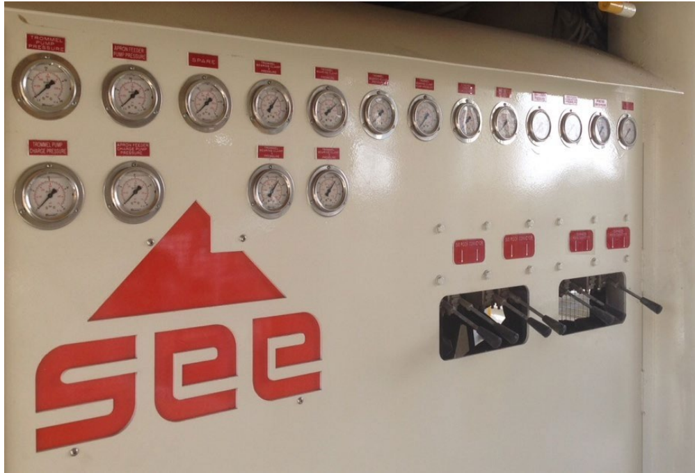
Diagnostic and Commissioning Panel
