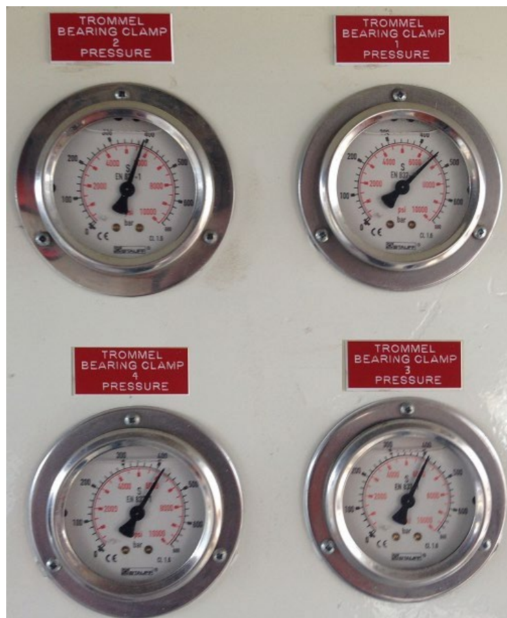
Trommel bearing clamp circuit gauges.
